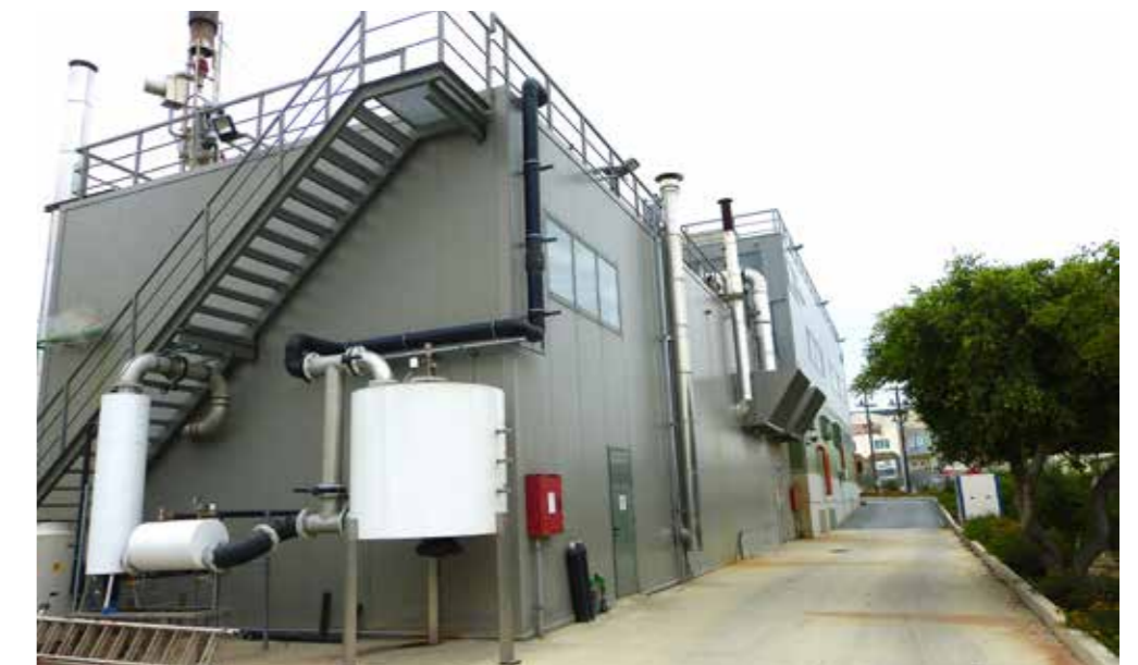
The Heraklion Biogas Plant features here in this part of the facility a special deodorization system that enables plant's integration into the urban environment and a highly specialized wastewater treatment system for the effluents avoiding any contamination of the environment.
