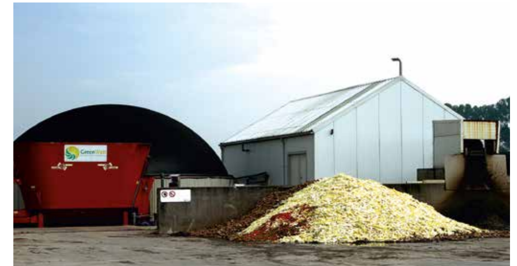
View of the Joluwa biogas plant. To the left the red receiving bin with the hydrolysis tank, the HYFAD unit is inside the shed. In the foreground the feedstock chicory roots and endive leaves alongside the solid digestate discharge. Further to the right, out of view, is the CHP unit and the post digester.
