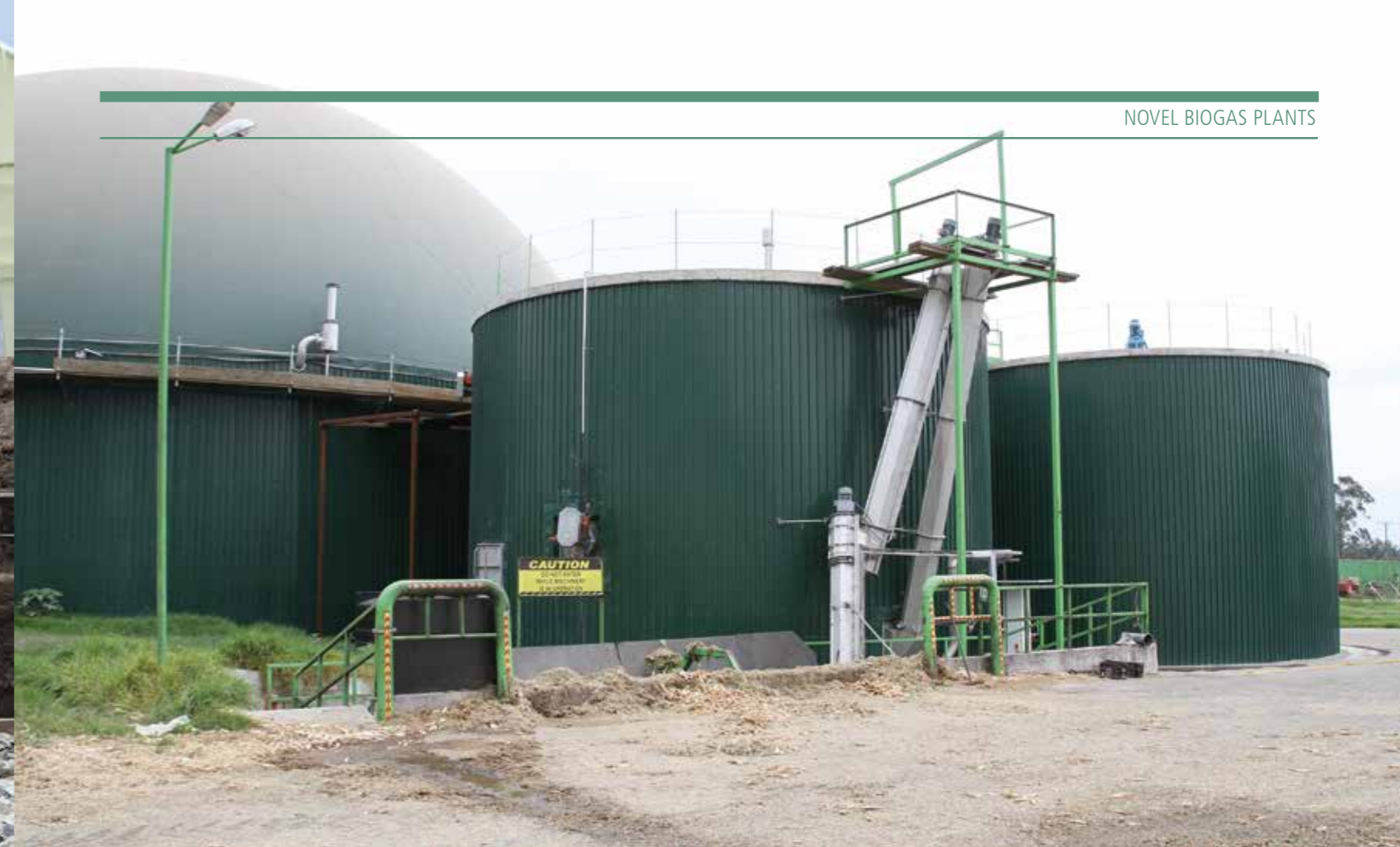
(Above) The biogas plant is a two-stage process type with a hydrolysis stage followed by the methanogenic stage.
