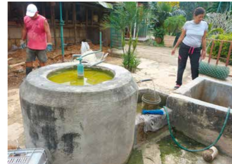
Top of the small scale biogas fermenter, which bottom plate is placed about 4 meter deep under the earth.
