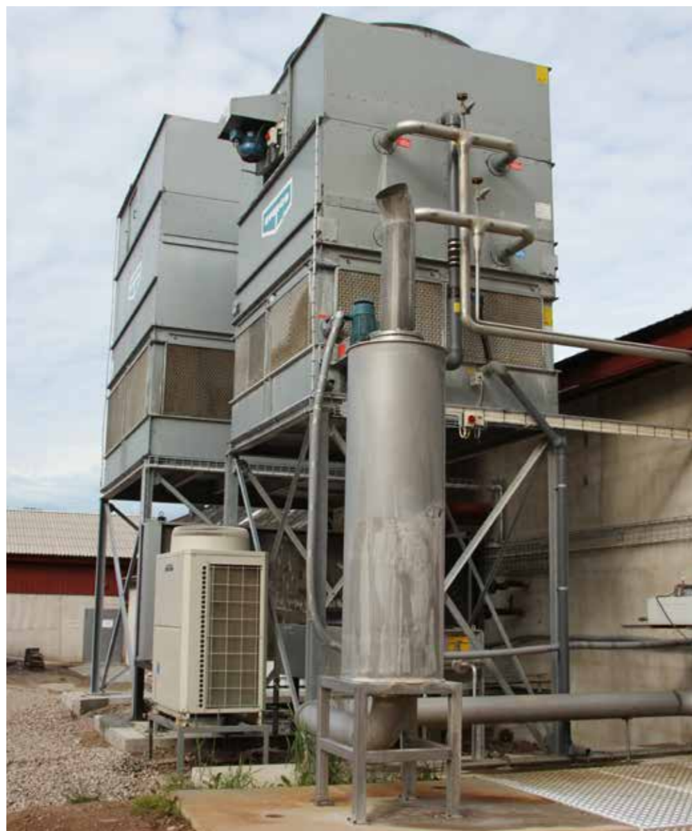
The CHP genset and ARP are located next to the dairy, a urea based agent is used to reduce NOx emissions.
