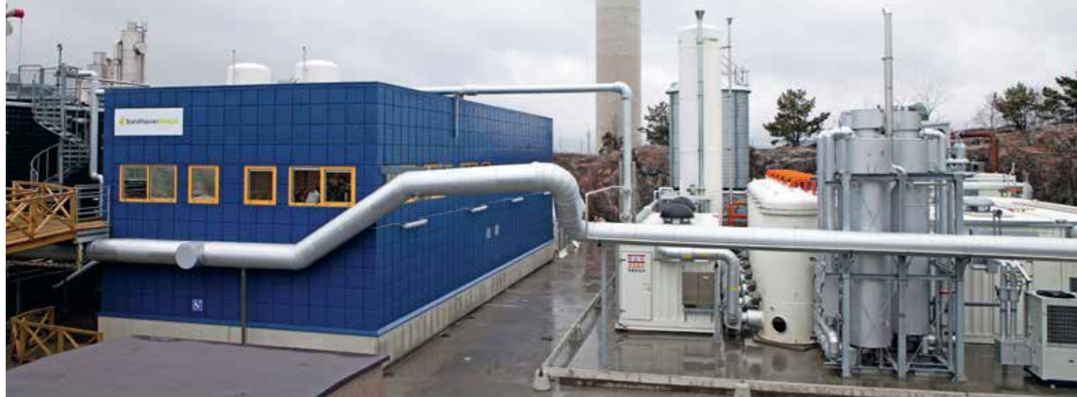
The investment in the new upgrading plant from Carbotech was SEK 93 million (≈ EUR 10 million) and the annual capacity is 125 GWh.
